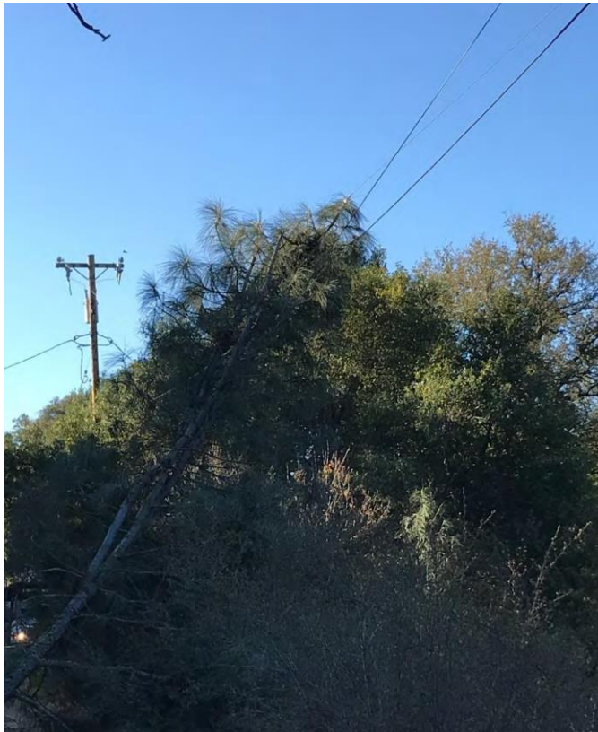
A tree blown onto conductors in unincorporated Lake County.
